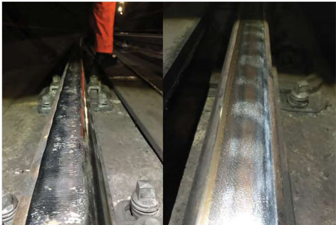
Figure 13: Rutting corrugation on modern track-form
